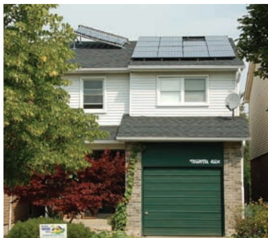
The West Toronto Initiative for Solar Energy (WISE) is one of the largest solar neighbourhoods in Ontario. ARISE was responsible for the supply and installation of all PV systems for WISE members. Currently, more than 30 PV systems are fully operational.
