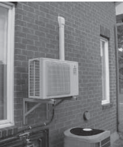
Mini-split system compressor (centre) installed at the CCHT Experimental House, pictured above a traditional ducted central air conditioner compressor.
