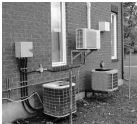
Efficient HVAC systems, such as a mini-split heat pump, contribute significantly to the energy performance of houses.
