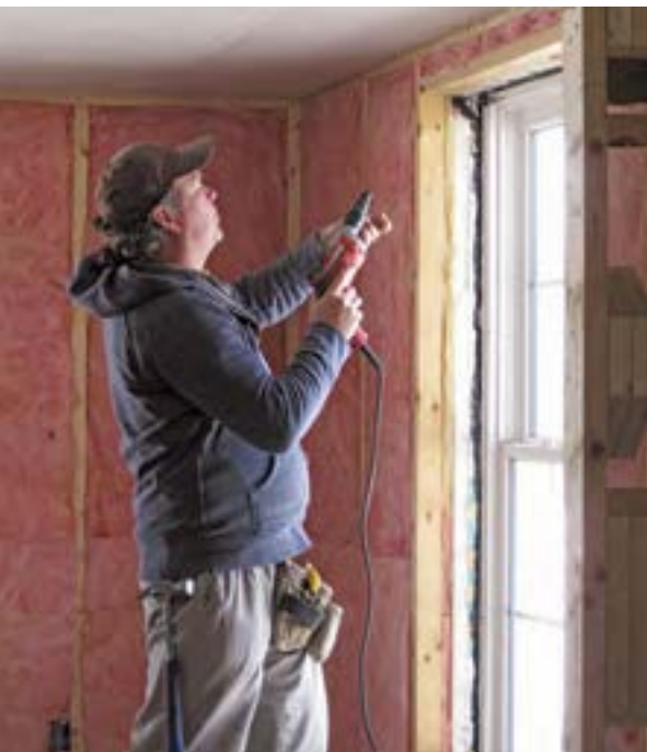
Built-up walls allowed insulation close to R40, with electrical, plumbing and mechanicals installed within a new non-structural wall cavity.
