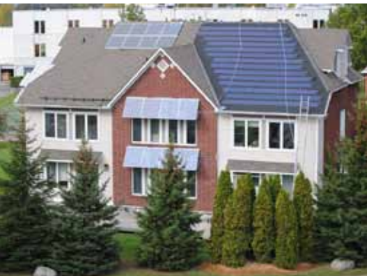
A roof-integrated photovoltaic system (right side of roof) was installed at the Canadian Centre for Housing Technology InfoCentre.
