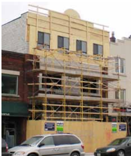
In this project on the Danforth in Toronto, the builder is renovating a main floor commercial unit with two floors of residential units above.
