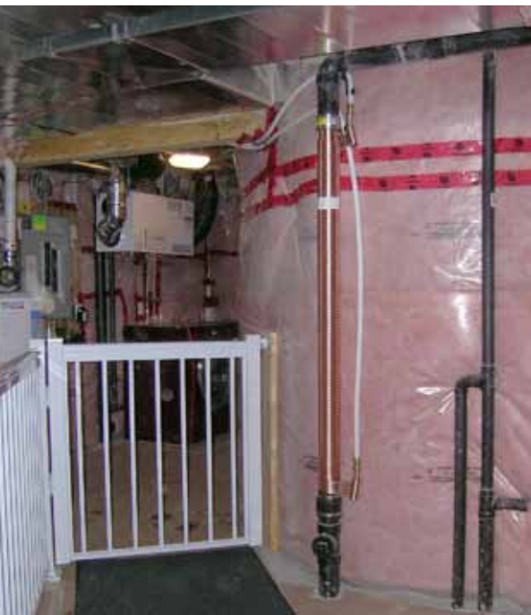
The Drain Water Heat Recovery Unit captures heat from showers, which in turn warms the home's cold water line to the hot water tank. This effectively reduces the energy required to warm the water in the hot water tank.
