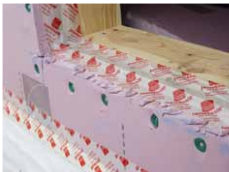
Increased air sealing details are incorporated to prevent air leakage in the home. This is achieved through Owens Corning's CABS system (Code Board Air Barrier System).
