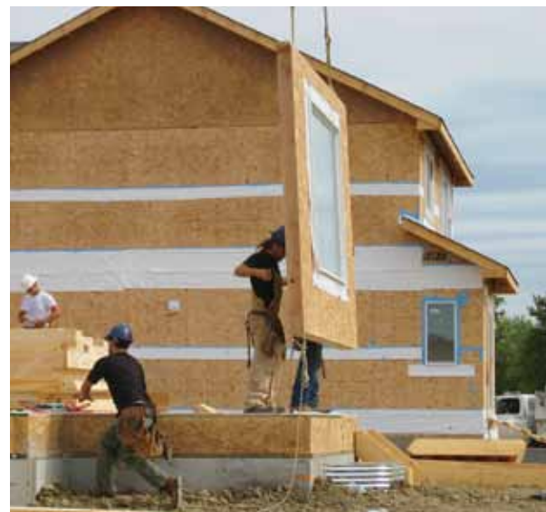
Panels built in the ACQBUILT manufacturing facility are assembled on site by a crew and the assistance of a crane.
