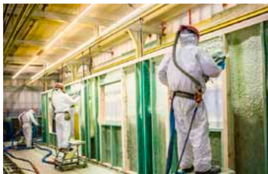
ACQBUILT employees install sprayfoam insulation, giving the home excellent thermal performance and a rock tight seal.
