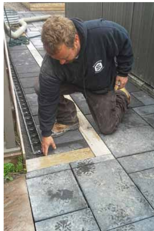
Ottawa-area contractor Adam Clark of Showcase Stone Works lays interlock pavers during a landscape renovation.
