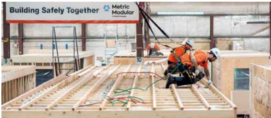
Metric Modular completes modular homes in a factory and ships them to sites.
